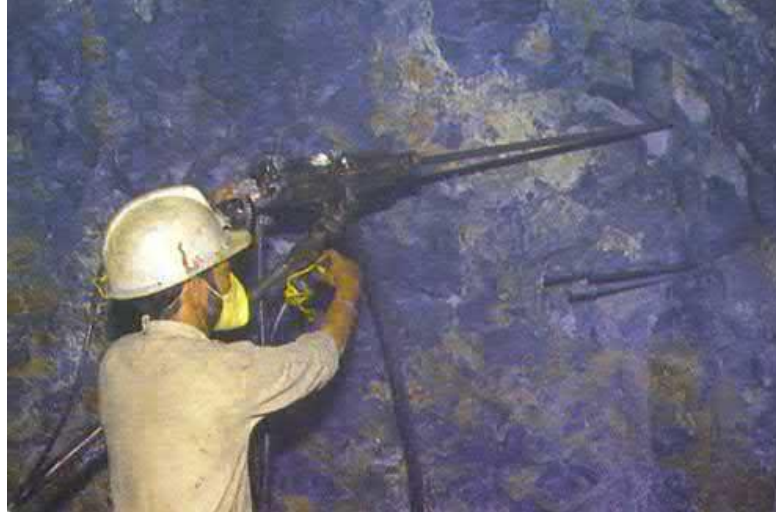
Figure7- Jackhammer drilling in rich sulfide mineralization for multipurpose use as underground mine face development and sample source for ore continuity and grade control.
